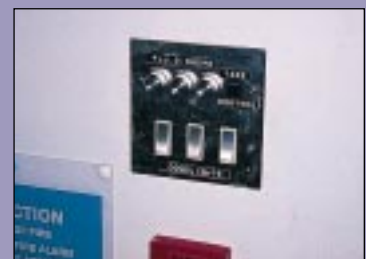
Note the clear and concise labelling of the building controls.
