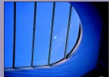
The rooflights above the stairs show a slight tendency towards air leakage.
