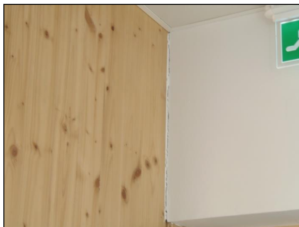
Figure 66: Crack in Wall Joint 2
