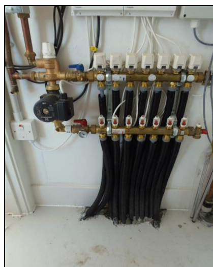
Figure 3: Manifold for under-floor heating
