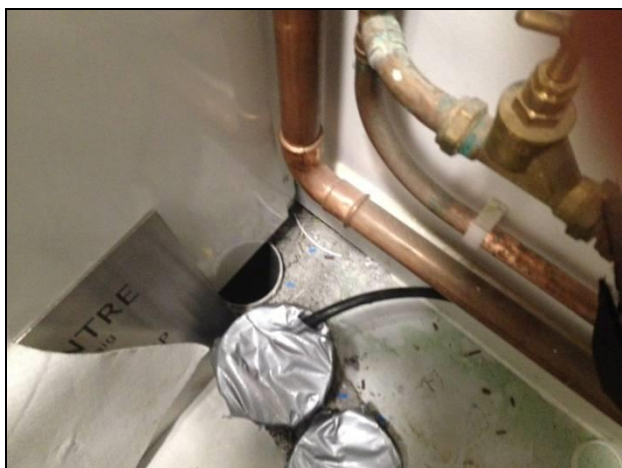
Figure 69: Open Pipe through Floor
