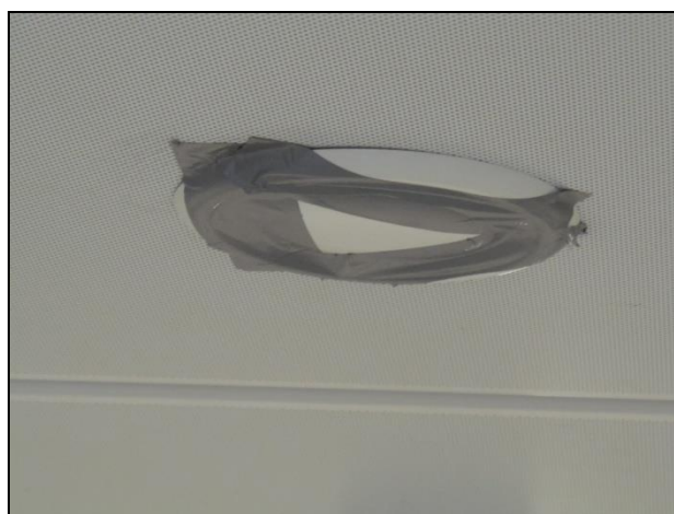
Figure 63: Sealed MVHR Vent
