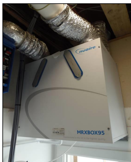
Figure 5: MVHR unit in plant room
