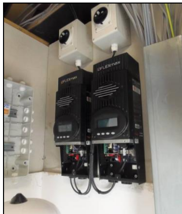
Figure 8: PV Charge Controllers
