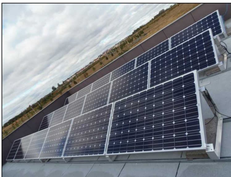
Figure 7: PV array on roof
