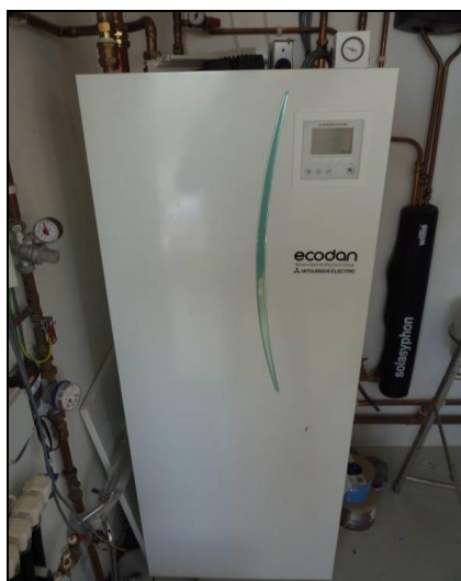
Figure 2: ASHP Cylinder Unit
