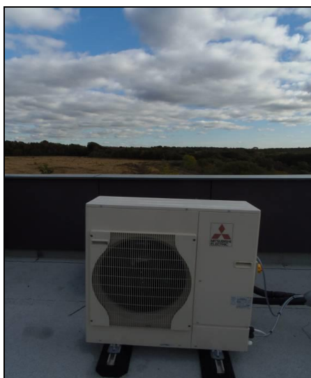
Figure 4: ASHP unit on roof
