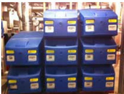
Above: Bank of condensing boilers to district heating system in rooftop plant room.
