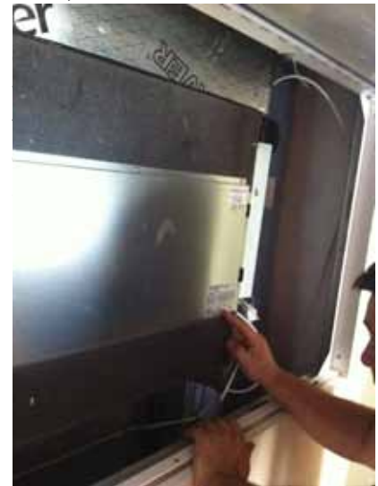
Above: In room individual air-handling units, vented to building facade and directly controllable by hotel guests.
