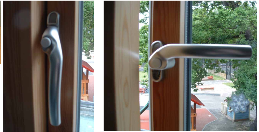
Fig 8.4.5 - Photographs showing the window handles with caps successfully installed. This system only worked with the side-hung windows.
