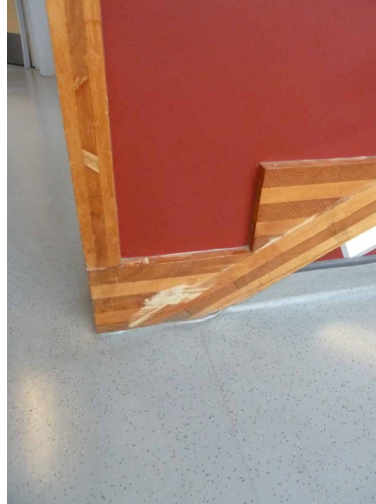
Fig.5.5.5- Defects in the manufacture of cross laminated timber were visible in some locations. The fire retardant coating caused the timber to yellow overtime, which was disliked by many.
