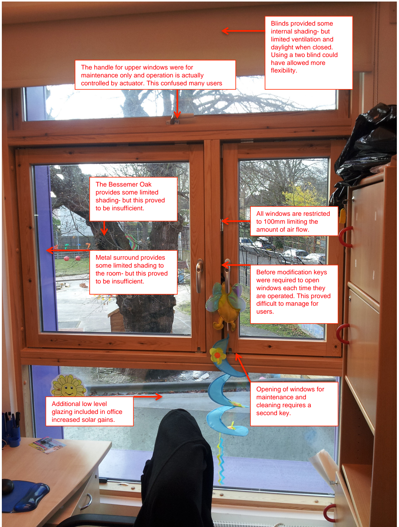
Fig.8.4.1 - New Building - first floor office window- a fairly typical arrangement of windows.
