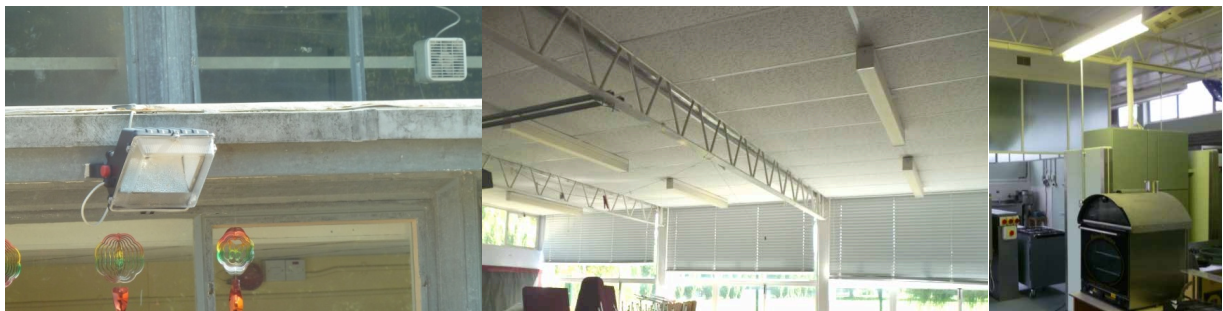
Fig 3.5.2 – Lighting in the Old Building - left: external Halogen Flood Light; middle: internal T5 lamps in classroom; right: T5 lamps in main kitchen
