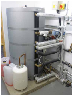
Fig.3.2.3 DHW calorifier located in the plant room of the New Building
