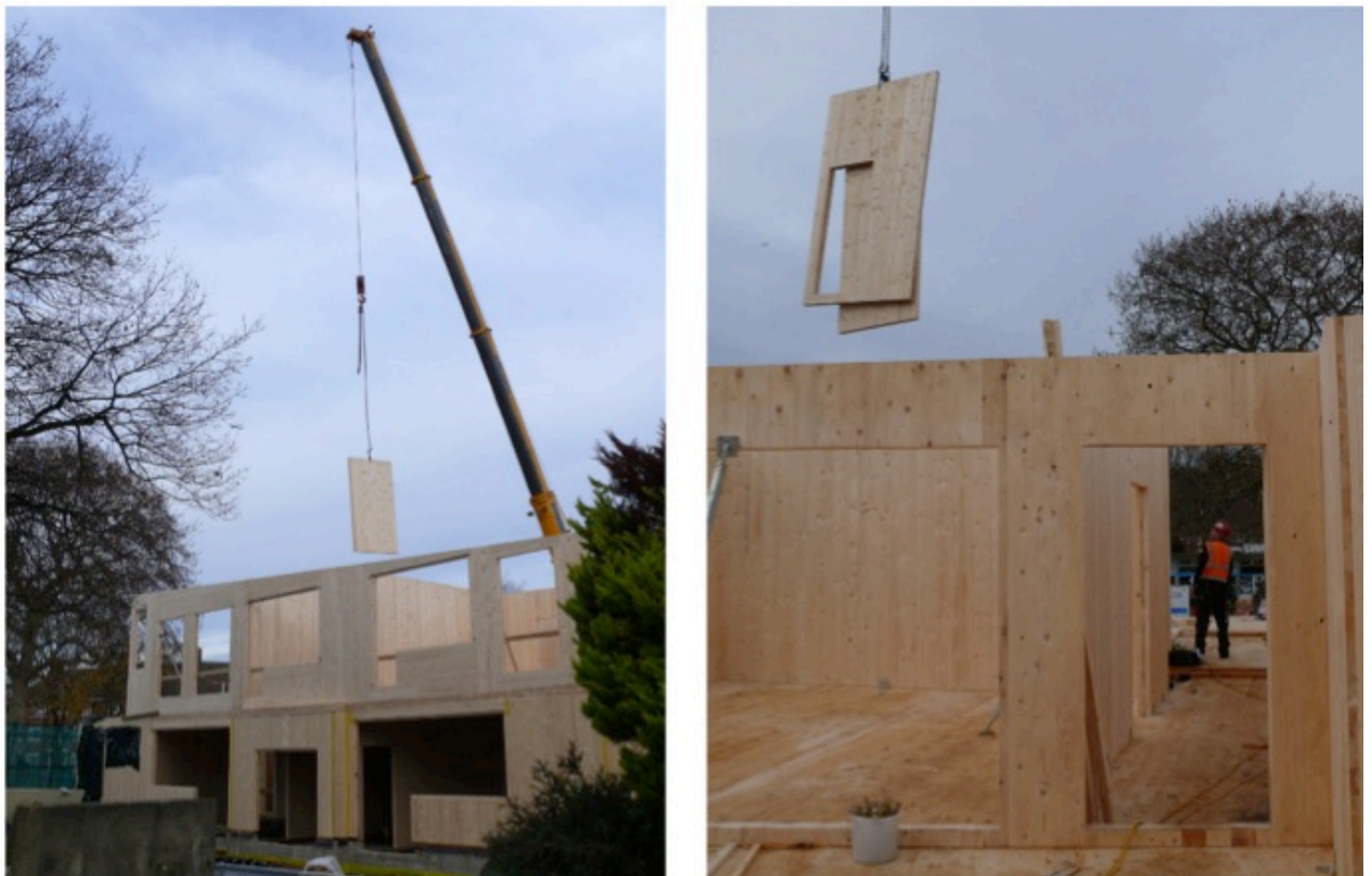
Fig 2.10.1 – Photographs showing the erection of the cross laminated timber frame in panel form. Due to off site manufacture the entire frame was erected in 10 days.
