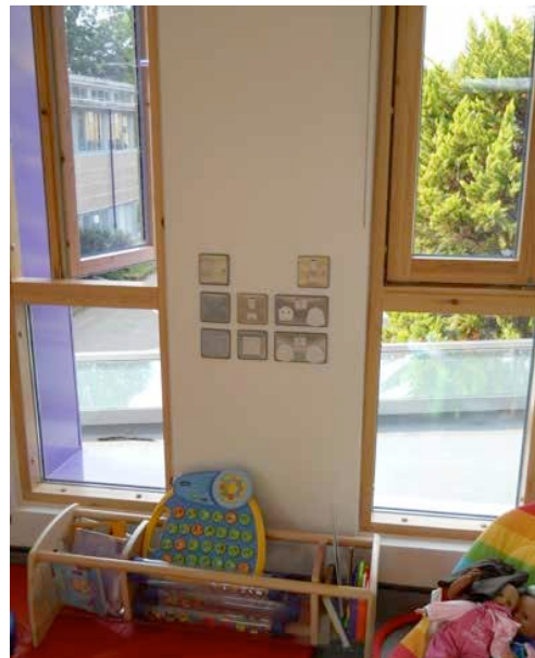
Excess of outlet sockets in the creche areas
