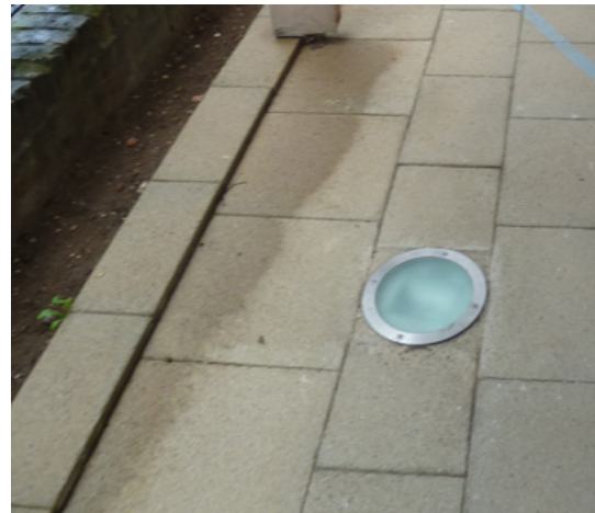
Fig.5.5.7 - Problems were experienced with external recessed lighting - with water leaking into fittings. These were replaced by the contractor but facilities staff complained future repairs would be expensive - they state a preference for wall mounted fittings with cheap replacement parts.
