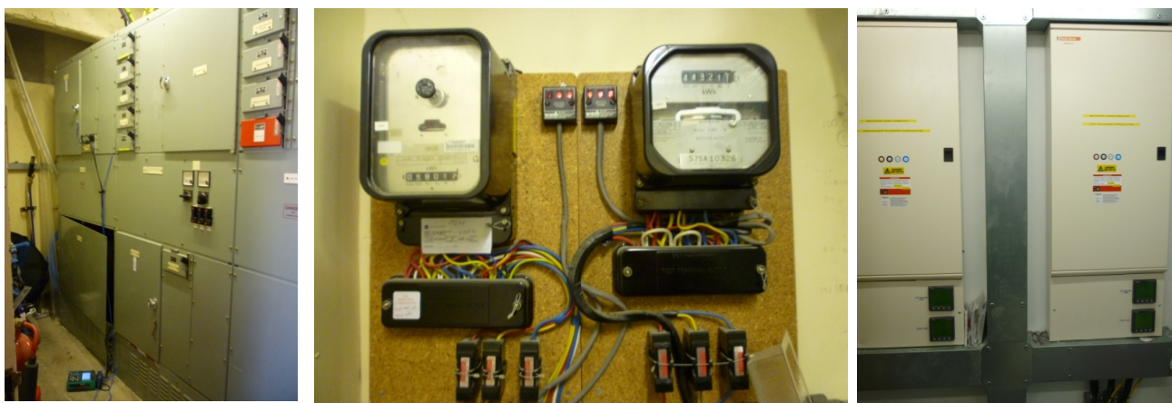
Fig 3.7.2 - Left: Electrical room in the Old Building; Middle: main utility meters in electrical room; Right: distribution boards in New Building plant room
