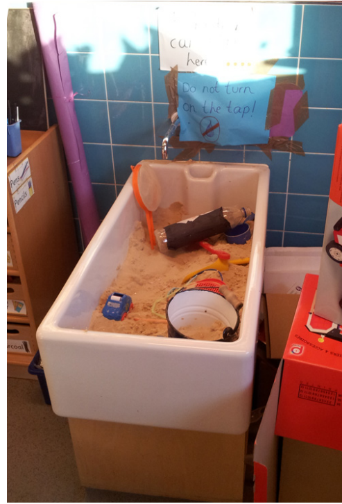
Fig.5.5.9 - Bespoke play sinks were fitted in the classrooms of the New Building. These were very popular with staff.
