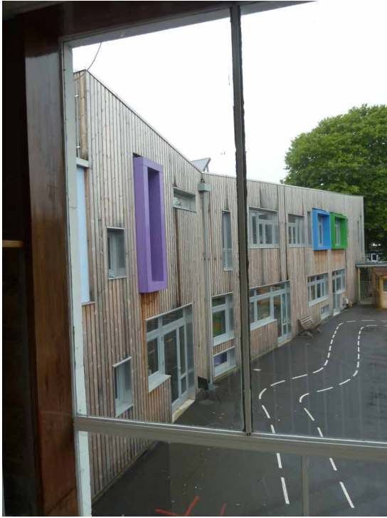
Fig.5.5.8 - Staining on the external cladding can be seen in vertical lines. This has been caused by water dripping from joints on the main capping. Remedial works were undertaken to improve this junction – however on future projects capping should have a greater fall toward the roof (away from the façade) and have a greater overhang to avoid this issue.
