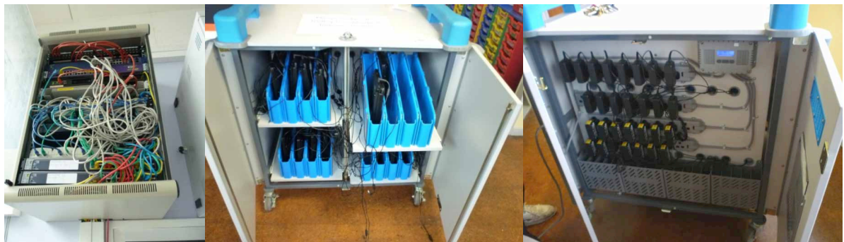
Fig 3.6.1 - Left: servers in ground floor circulation corridor, middle and right: Portable laptop charging stations
