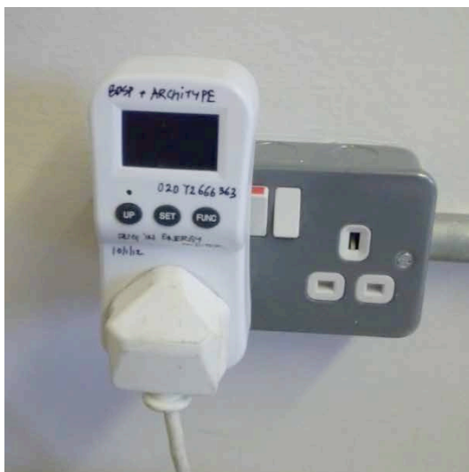
Fig.6.2.1 - Photograph of a portable plugin meter used to help the BPE team calculate electrical loads for electrical equipment as part of the TM22 analysis.
