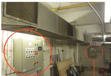
Main Control Panel
