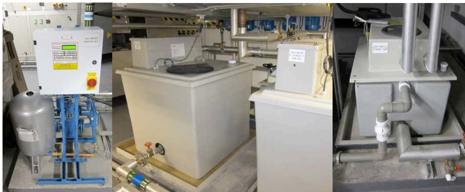
Figure 3-17 Cold water booster set; cold water storage; rainwater break tank
