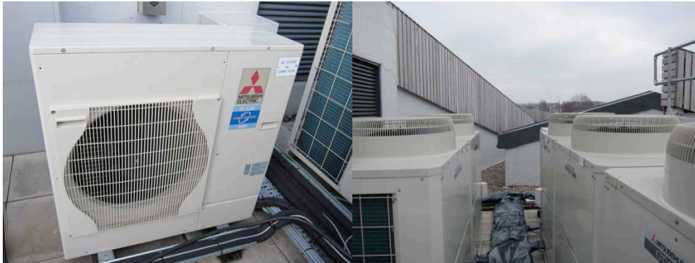
Figure 3-7 Comms heat pump; Outdoor units for underfloor distribution system
