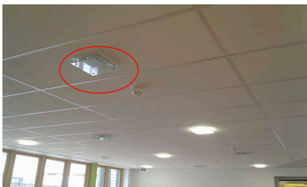
Figure 7-3 Disconnected lights in GF43
