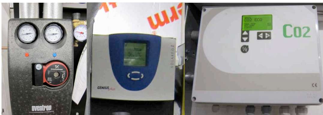
Figure 3-15 Analogue gauges with solar thermal pump; solar controller; heat pump controller
