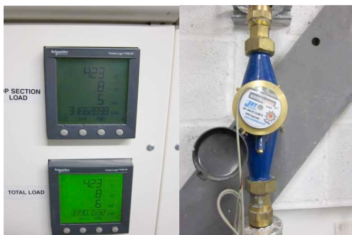
Figure 3-19 Distribution Board submeter (l); rain water meter (r)
