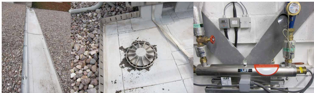
Figure 3-18 Rainwater channel on roof; rooftop drain to below ground rainwater storage tank; rainwater UV purification
