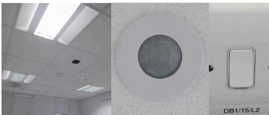
Figure 3-3 T5 lighting; PIR sensor; typical light switch
