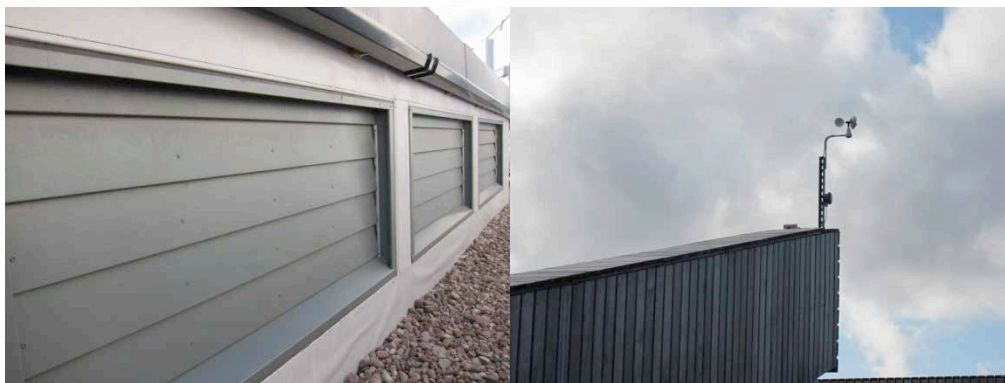
Figure 3-4 Mechanically actuated louvres; wind speed and external temperature sensors
