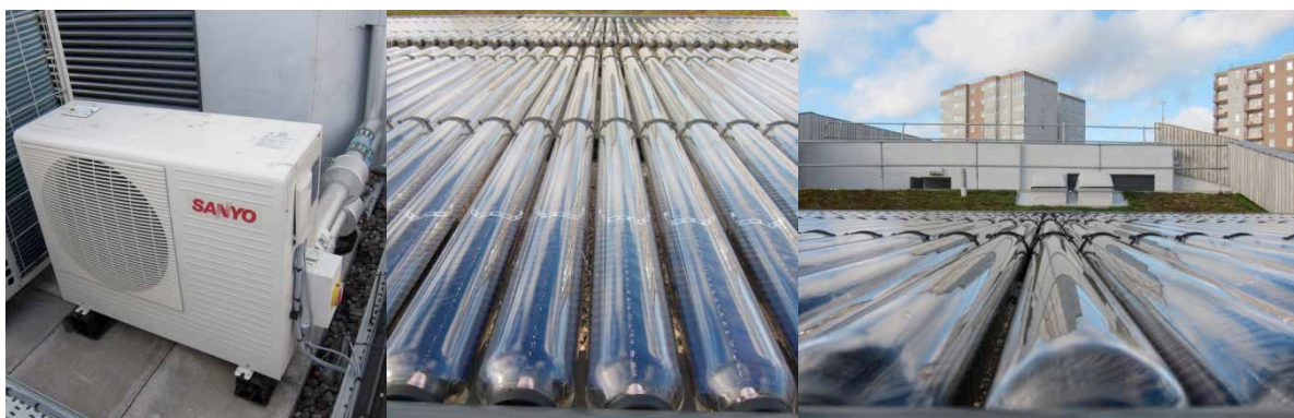
Figure 3-14 Dedicated DHW heat pump (I); Solar thermal installation
