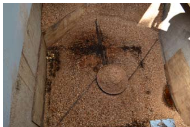
Figure 7.3: Moisture issues in the fuel store
