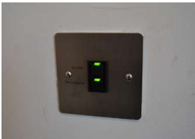
Figure 7.5: Classroom lighting controls. ‘Whiteboard’ switch could be misunderstood
