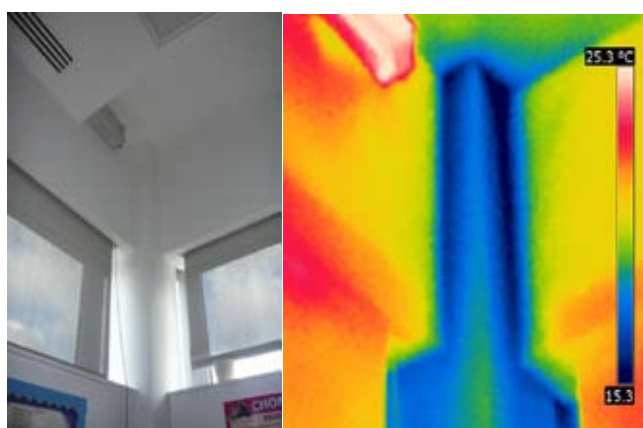
Figure 7.1: One of the few thermal bridges identified
