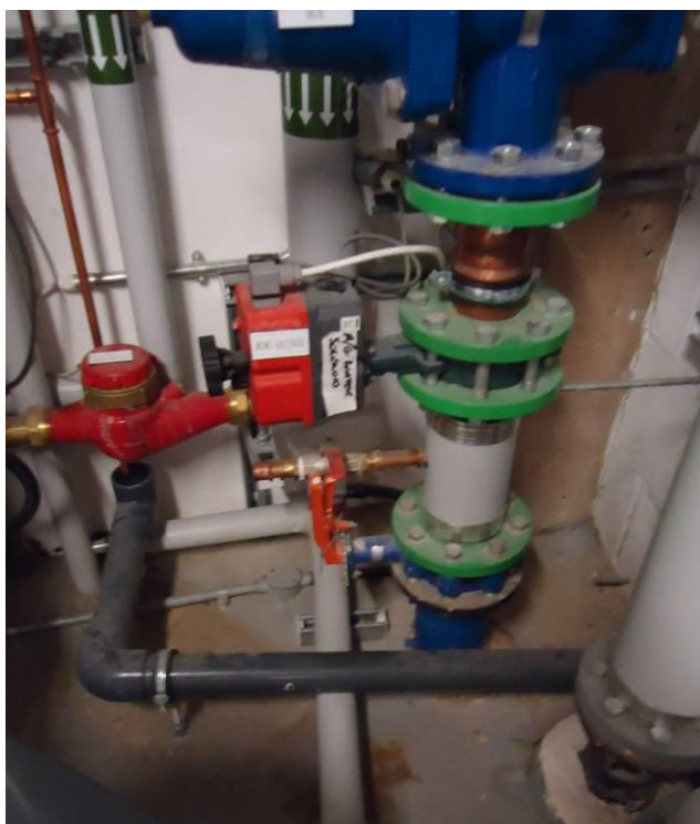
Figure 10.38. Location of incoming cold water supply pipes close to heating flow and return pipes in plant room Faraday block. This could possibly be the cause of the elevated cold water supply temperature.
