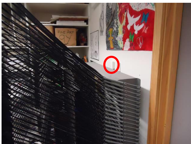
Figure 3.9. CO 2 sensor on wall in room L210 Cade North block highlighted in red, obscured by general clutter.
