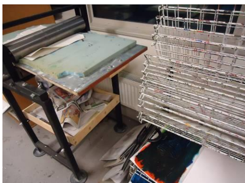
Figure 7.9. Radiators in L210. Art room Cade North obscured by various equipment.
