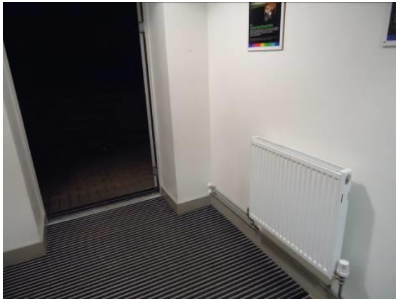
Figure 7.10. Door to outside in Sports block. Observed during several site visits to be left open for much of the day even though the heating is on.
