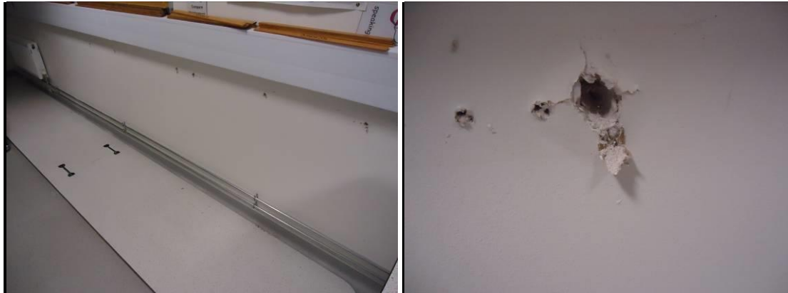
Figure 10.16. Fallen bench in Science Opportunity Centre in Faraday block.
