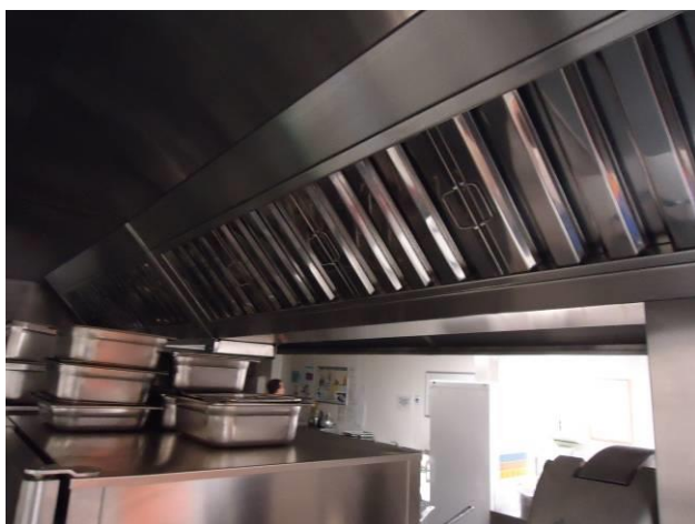
Figure 10.40. Kitchen extract fan which is on continuously throughout the day.
