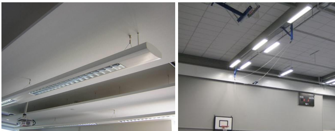
Figure 3.1. General electric lighting installed in classrooms (left) and Sports Hall (right).
