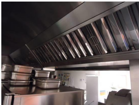
Figure 6.34. Kitchen extract which was observed to be running continuously.
