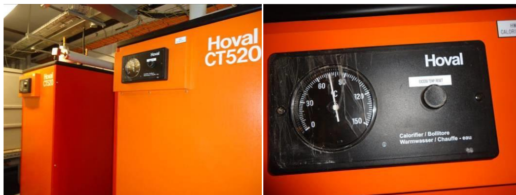
Figure 10.31. 2 No. Hoval calorifiers in Austen block plant room and temperature dial on one. Note the temperature is being kept over 75°C.
