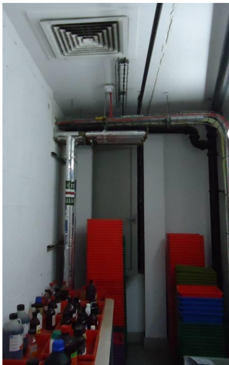
Figure 10.46. F201 Chemical store Faraday block, note open night vent and mechanical ventilation panel which was extracting.
