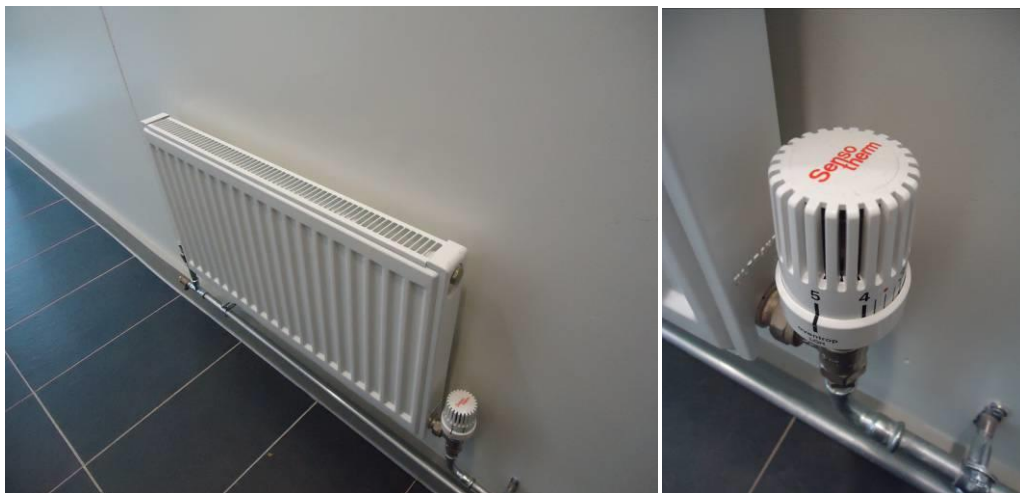
Figure 10.29. A radiator in a circulation space. The TRV was set to maximum of '5', which was typical for many radiators in circulation areas.
