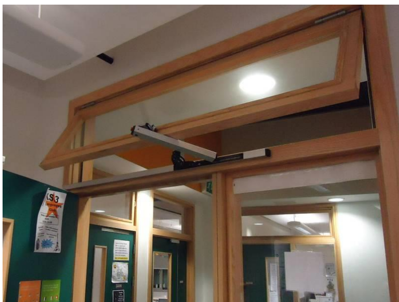
Figure 10.35. Fanlight vent above door leading to corridor in open state.
