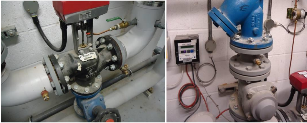
Figure 10.19. Un-insulated pipe joints in Faraday block plant room.
