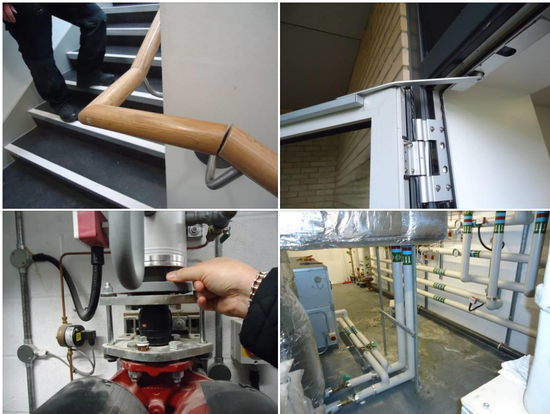
Figure 10.17. Clockwise: Loose hand rail, bent door opener, loose bolts on pump fitting, and floor damage from burst water pipes in plant room.
