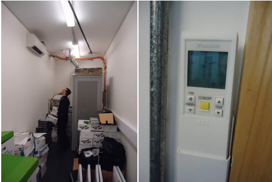
Figure 7.14. Small server room in Tenzing block and 18°C set point.
