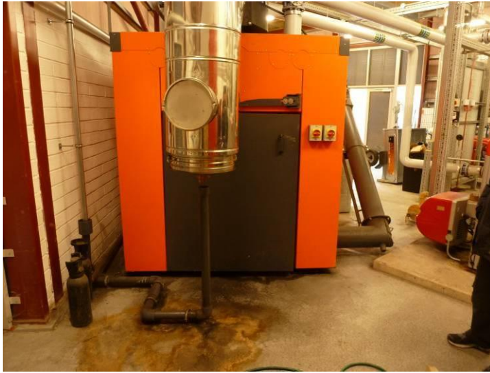
Figure 10.47. Biomass boiler, note the stain on the floor in front of the boiler indicating blow back.
