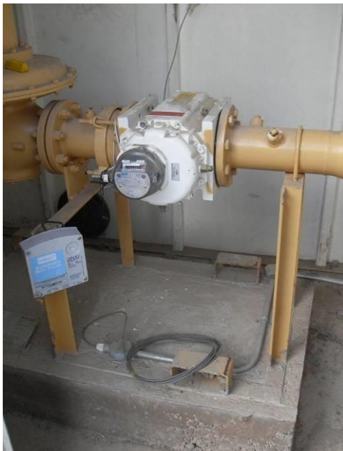
Figure 10.8. Site (north) fiscal gas meter with fiscal datalogger wired and the unterminated BMS data cable.
