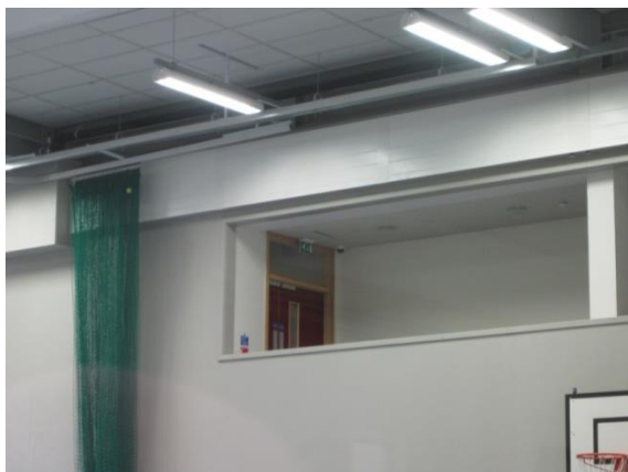
Figure 3.4. High level radiant panels in the main hall in the Sports Centre.
