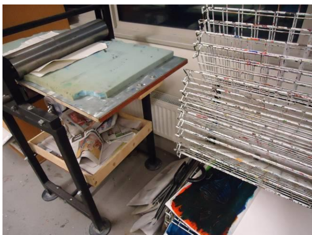
Figure 10.30. Radiators in L210 Art room Cade North obscured by various equipment.
