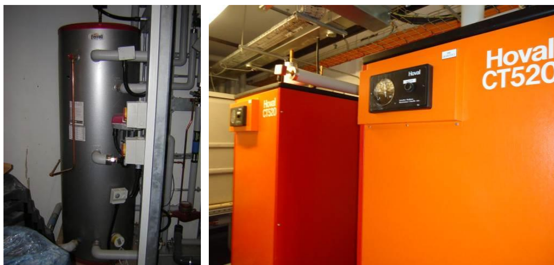
Figure 3.5. Storage calorifier in the Faraday / Austen plant room (left) and Sports Centre plant room (right).
