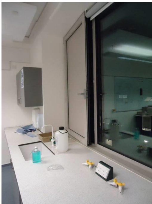
Figure 10.33. One of the night vents left open in F210 Faraday block while extract ventilation left on high.
