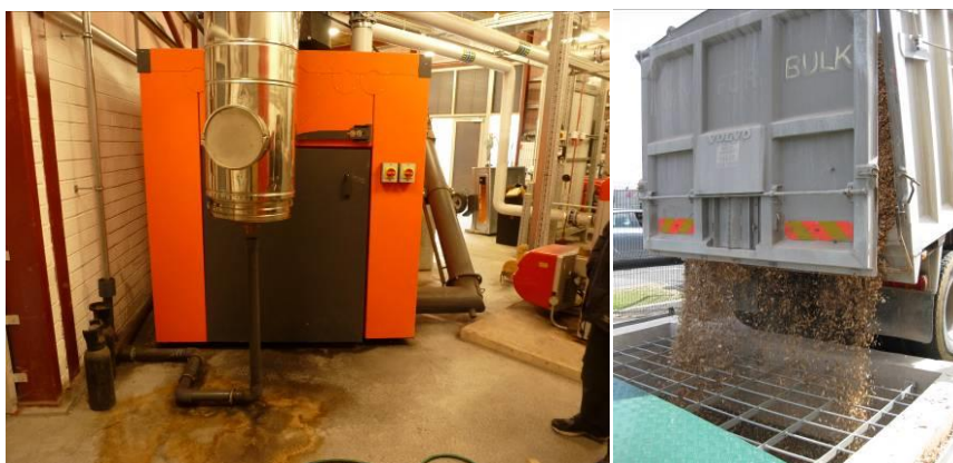
Figure 7.2. Biomass boiler (left) with the stain on the floor in front of the boiler indicating blow back and biomass delivery (right).
