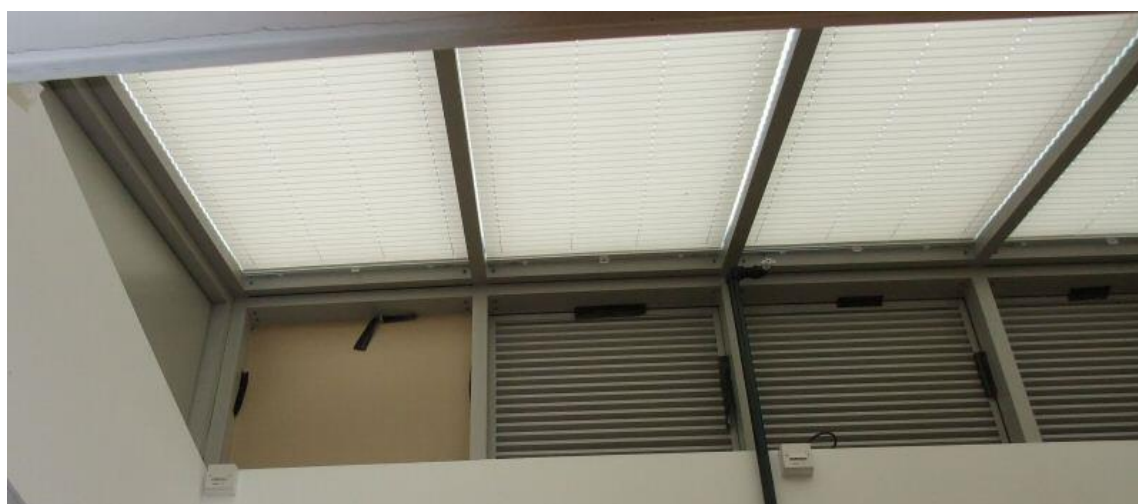
Figure 10.9. High level mechanically actuated vents in room L222 / L226, with evidence of them having been blocked up and isolated using local switches when building in summer control mode during the winter as a result of failure of the controlling PC.
