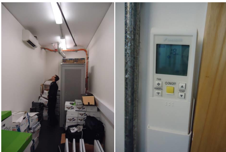
Figure 10.43. Small server room in Tenzing block and 18°C set point.
