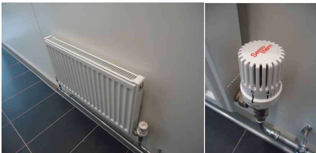
Figure 7.8. Radiator in circulation space in Austen block. TRV was set to maximum of 5, which was typical for many radiators in circulation areas.
