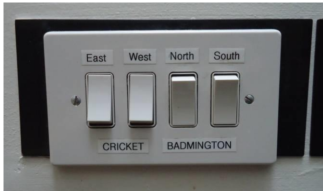
Figure 6.27. Light switch for Sports Hall located in reception area.
