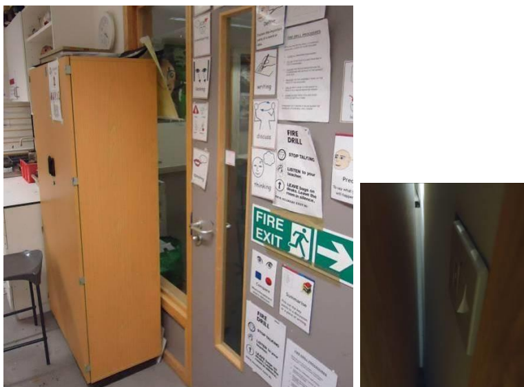
Figure 7.11. Light switch in classroom obscured by cupboard.
