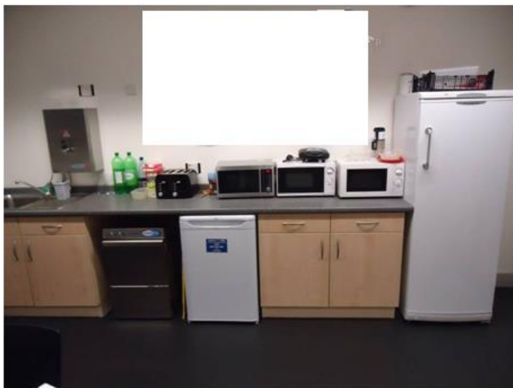
Figure 10.27. Kitchen appliances in Tenzing's Staff Room. These are all wired into supplies monitored by the Power submeter.
