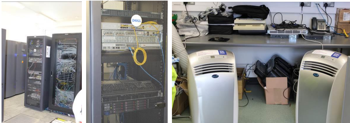
Figure 3.10 IT Server Room and IT workshop
