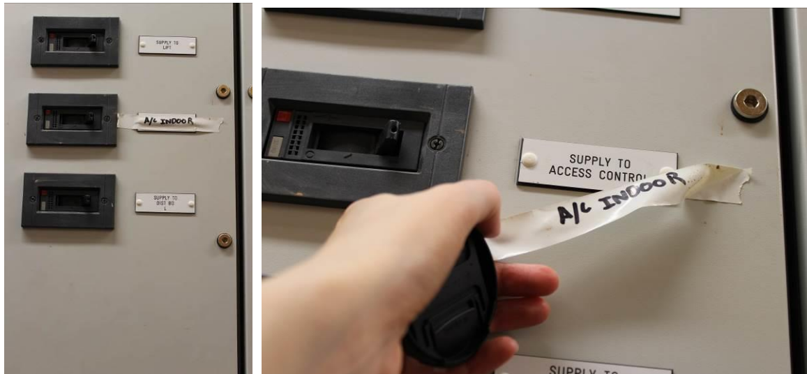
Figure 7.30 Images of A/C indoor duct tape notice over Access Control Label.
