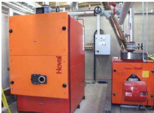
Figure 3.1: Biomass Boiler and Oil Boiler
