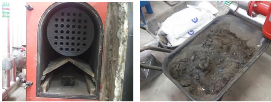
Fig 6.1 Biomass Boiler Maintenance
