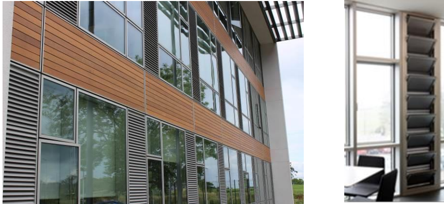
Figure 3.6 Automatic Vents Inside and Out
