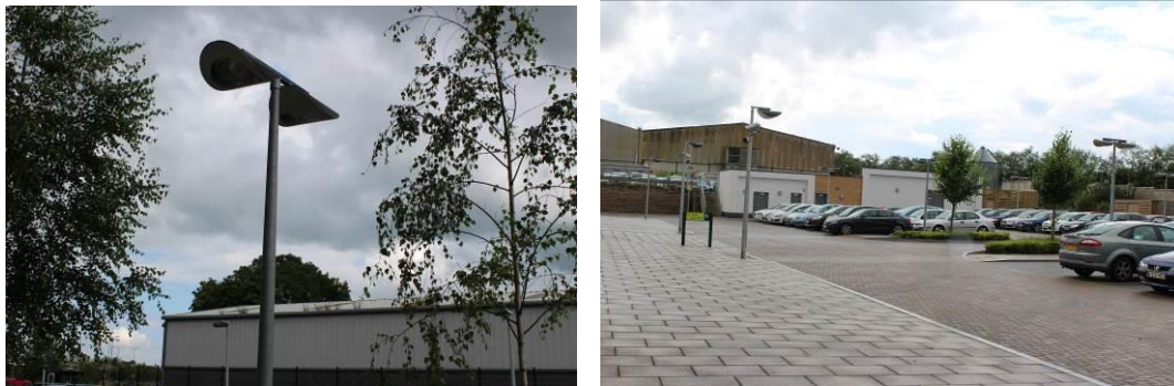
Figure 3.9 External lighting in the car park
