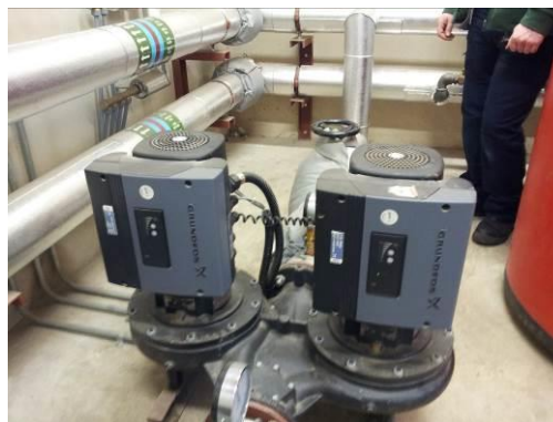
Figure 3.2 Pumps for Heating System
