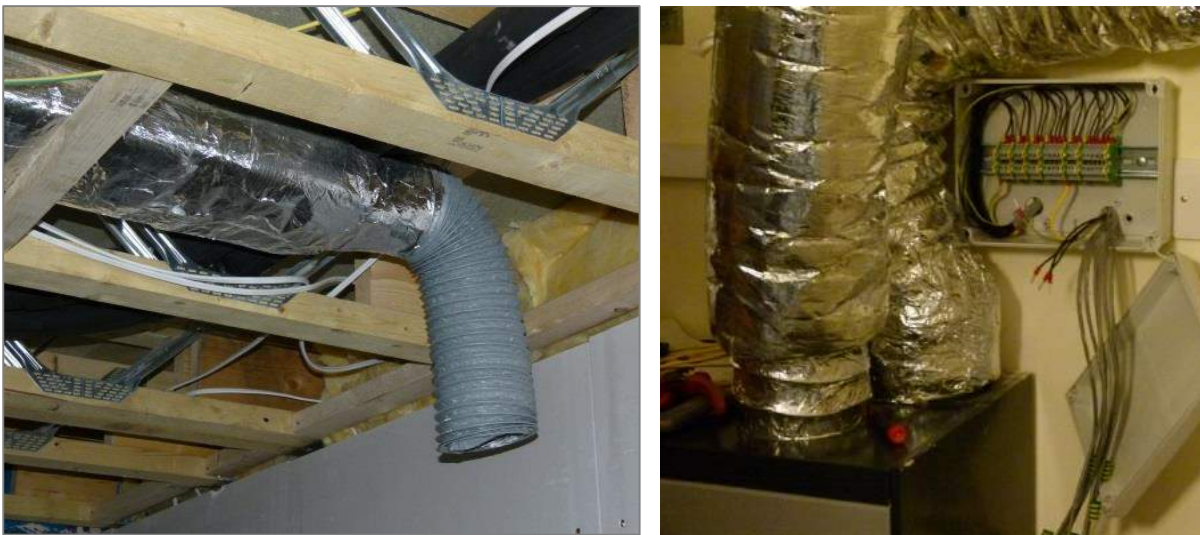
Figure 6.3b. Rigid rectangular ducting and flexible ducting to MVHR unit. Panflex acoustic attenuators employed.
