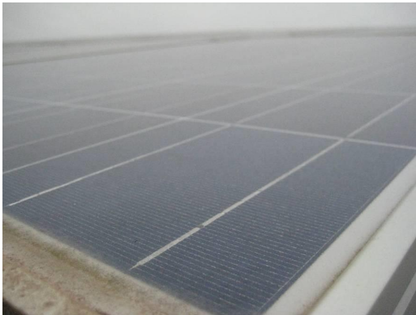
Figure 6.19: PV array on roof of NCC. Note the dirt covering the panels which will reduce the performance.
