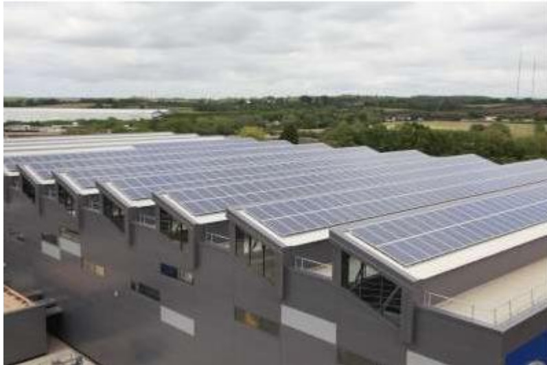
Figure 3.4: Photovoltaic array mounted on the roof of the NCC.
