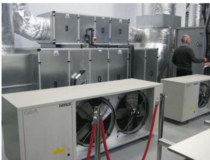
Figure 5.3: New clean room AHU unit inside the Main Workshop.
