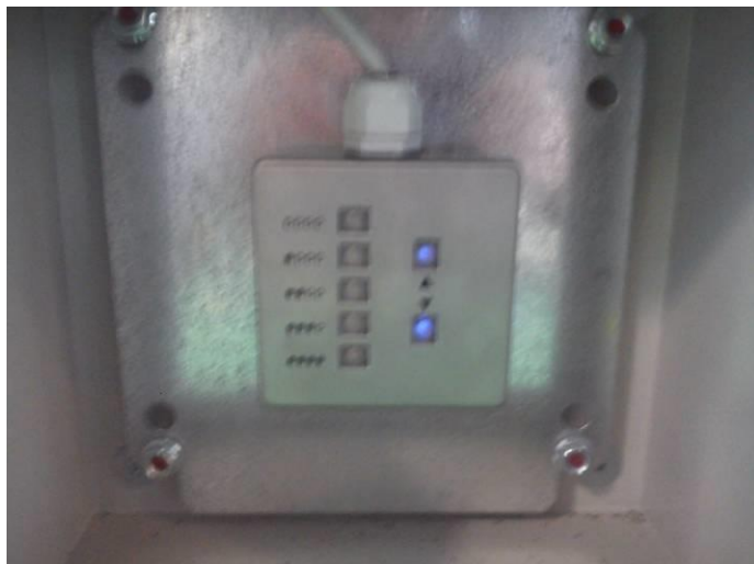
Figure 3.1: Manual lighting control for the workshop area.
