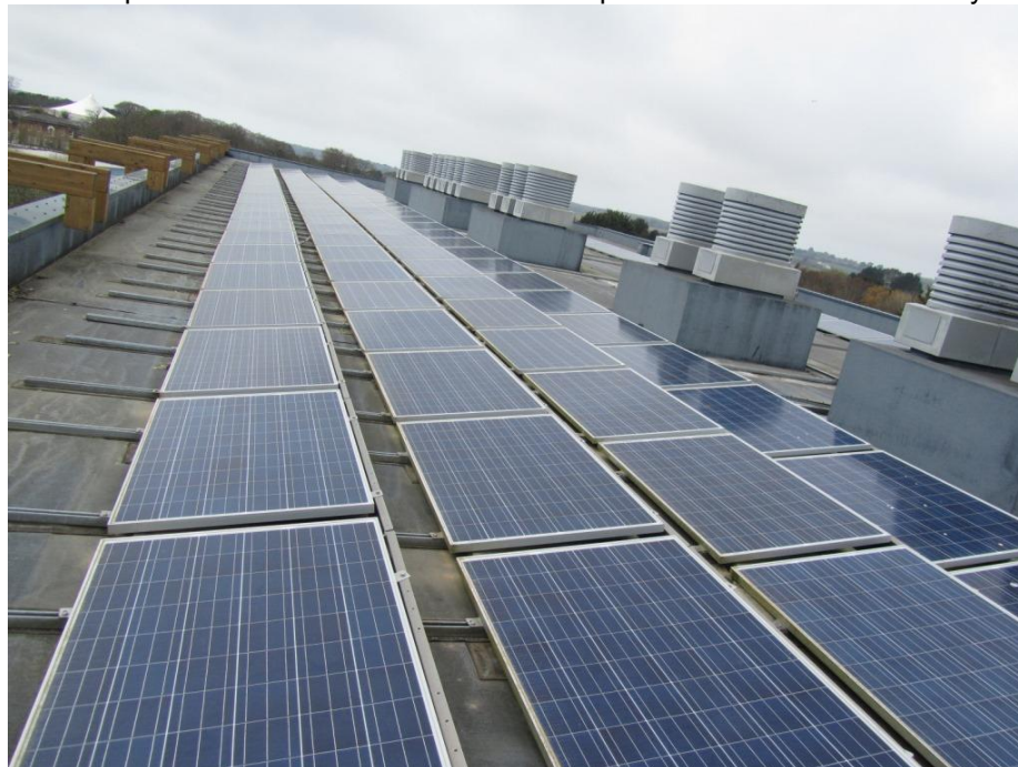
Figure 6.9: PV arrays installed on the roof (maximum design power output: 28.2 kWp)
