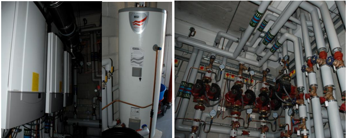
Figure 19 The plant room contains three wall-hung gas boilers as back-up.
