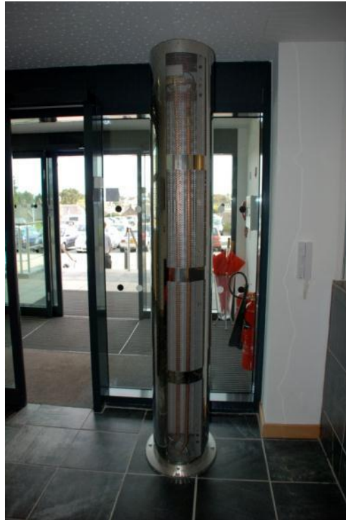
Figure 10 Unused air curtain
