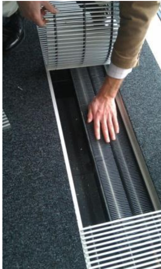
Figure 31 Trench heaters in meeting rooms
