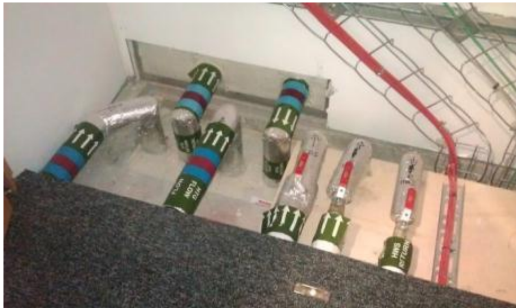
Figure 6 Under-floor services visible in a riser access cupboard
