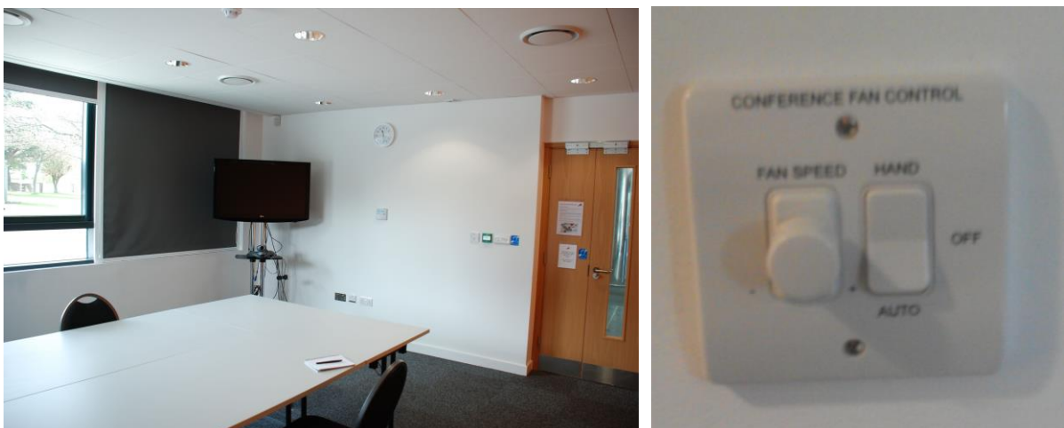
Figure 20 Air-conditioned meeting room and conference room fan controls
