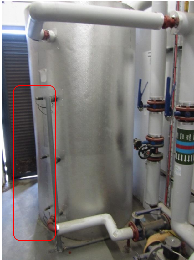
Figure 6.16: Shortcomings in biomass buffer vessel insulation can lead to high standing loss
