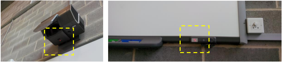
Figure 7.4 ground floor workshop projection board on standby
