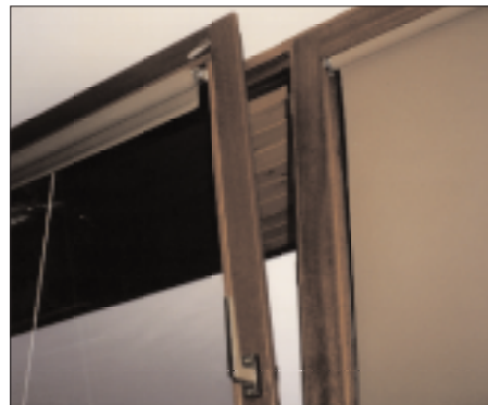
Windows, blinds and solar shielding
