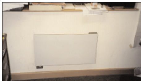
Perimeter electric heaters
