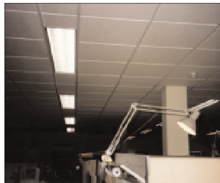
Ceiling and task lighting
