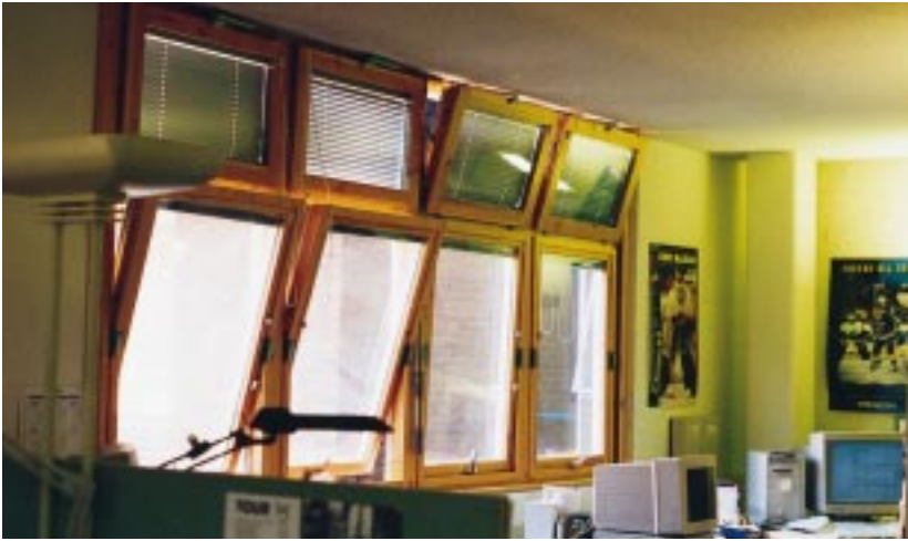
Figure 17 Uplighting on when the blinds are partially closed
