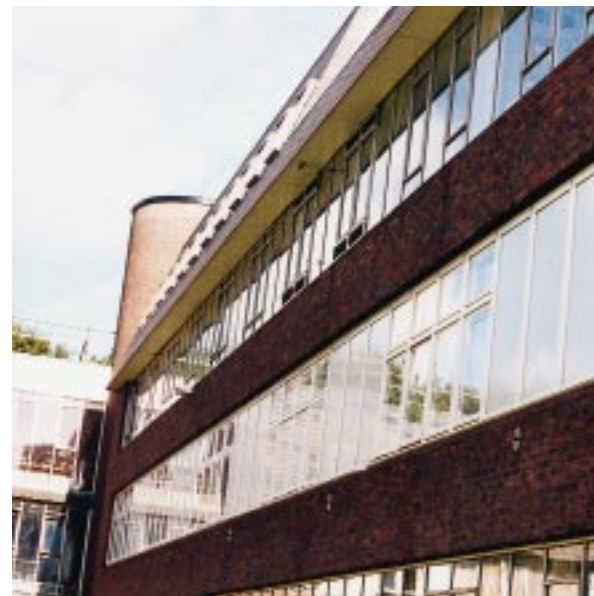
Figure 4 The new window system is the principal element in the refurbishment of the design studio on the first floor. It optimises the glazed area, in this case by halving it, and is triple glazed to reduce heat loss. Mid-pane venetian blinds control solar heat gain and glare, and incorporate a remotely operated 'hopper' window, which opens inwards, for secure cross-ventilation and night ventilation.
