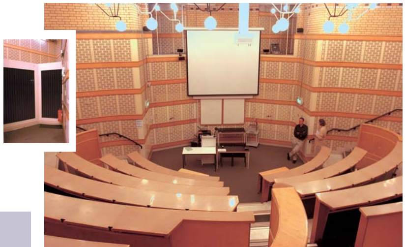
Auditorium 1.10 is the building's flagship space. The natural ventilation works well, with heat accumulating at high level and exhausting through two chimney stacks behind the screen. For auditorium 1.12, the heating coils set in the external wall (inset) are unable to raise the temperature of incoming air winter.
