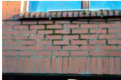
Figure 8. Clay bricks deteriorating.
