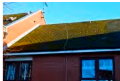
Figure 9. Moss growth on concrete tiles.
