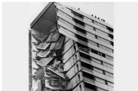
Figure 15. Ronan Point, progressive collapse (Sources: https://buildingfailures.wordpress.com/1968/02/06/ronan-point-disaster/ ).
