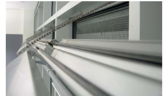
Above and top: City Academy windows and actuators
