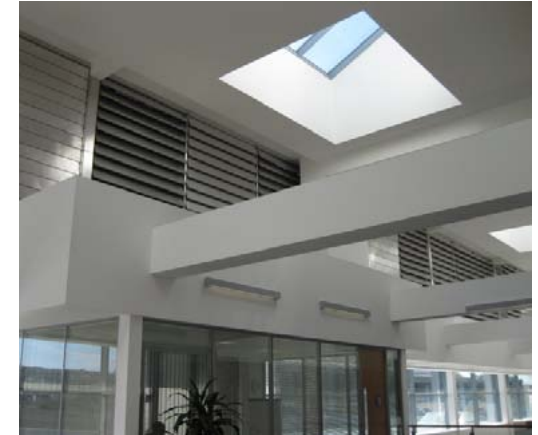
Ceredigion atrium showing the motorised louvres in the atrium (at high level)
