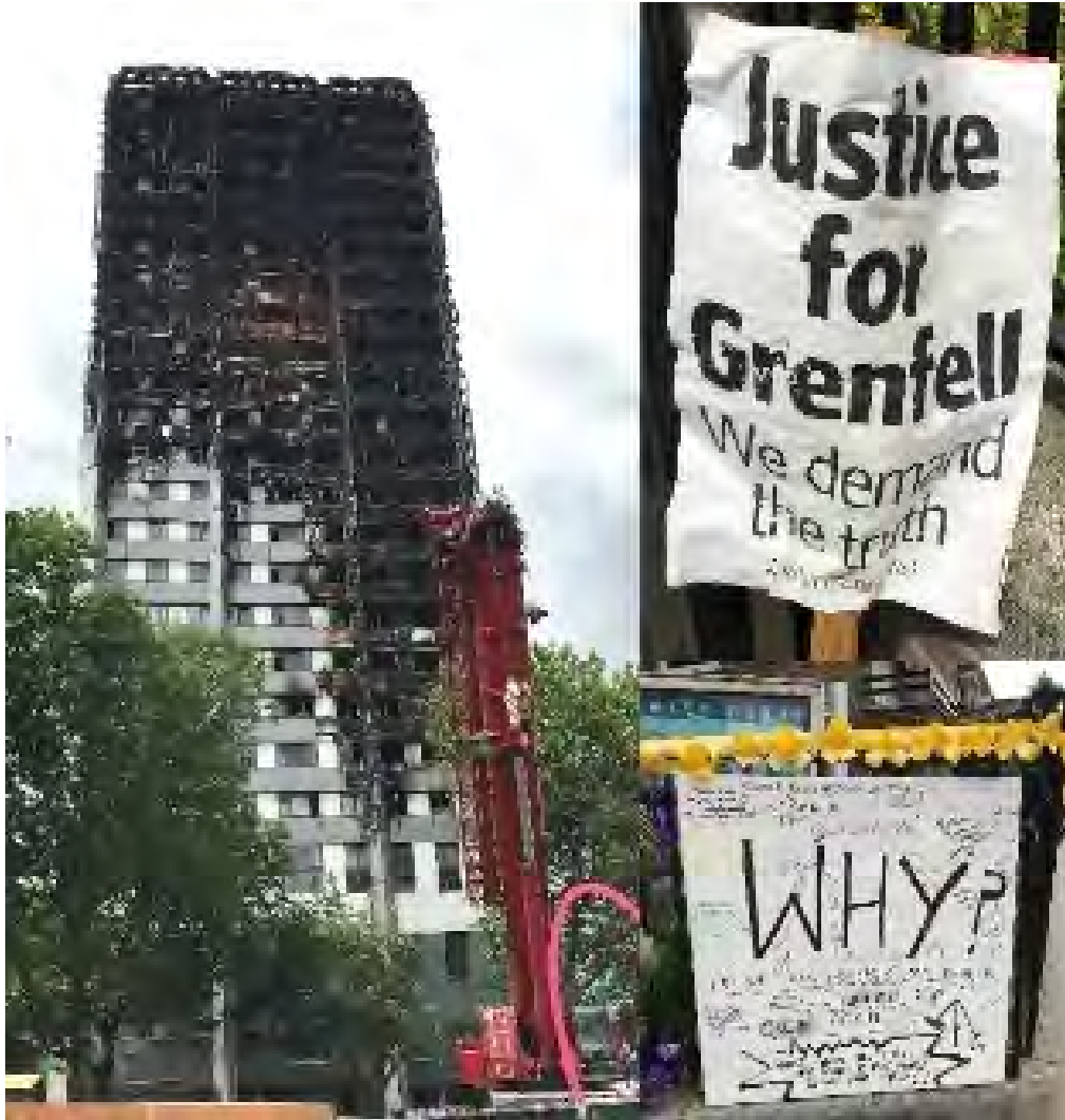
Figure 7. The devastating fire in Grenfell Tower in London, which cost 72 lives, was fueled, in part, by the same components we seek to improve thermal performance and reduce energy use in buildings. What can we learn from this? Photo: D.J. Lemieux
