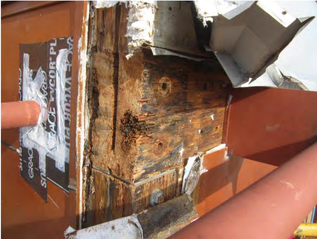
Figure 6. Moisture ingress and decay in a typical engineered wood structural member. Photo: Wiss Janney Elstner, Inc.
