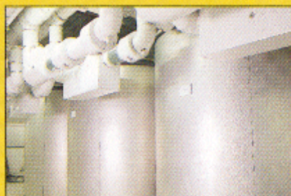
Planning restrictions on height led to the use of ice storage at 1 Aldermanbury Square.
