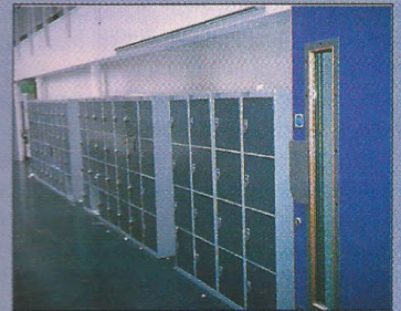
Student lockers in the circulation corridors, added after handover, are causing increasing congestion.
