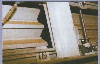
The roof-level ventilation dampers were found to be very leaky along the top and bottom blades.
