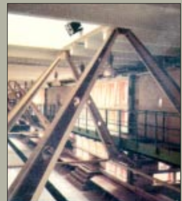
De Montfort: the striking characteristics of the high-bay SON lamps do not encourage frequent manual switching.
