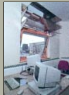
At APU, the twin internal light shelves of semi-transparent reflective glass have proved ineffective in enhancing light levels deep into the space, as the daylight is reflected into the coffers of the waffle slab ceiling.
