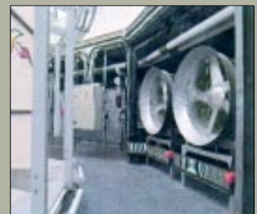
Heat recovery means constant system pressure drops at Tanfield House.
