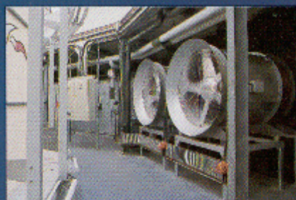
Filters and heat rejection coils in the extract system always mean high pressure drops.
