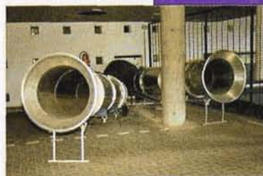
Two of the three medium BREFANs set up in the basement car park of the Enschede Tax Office extension.
