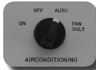
Figure 5: Wall-mounted rotary switch accessible to all users controlling the air conditioning and ventilation systems.
