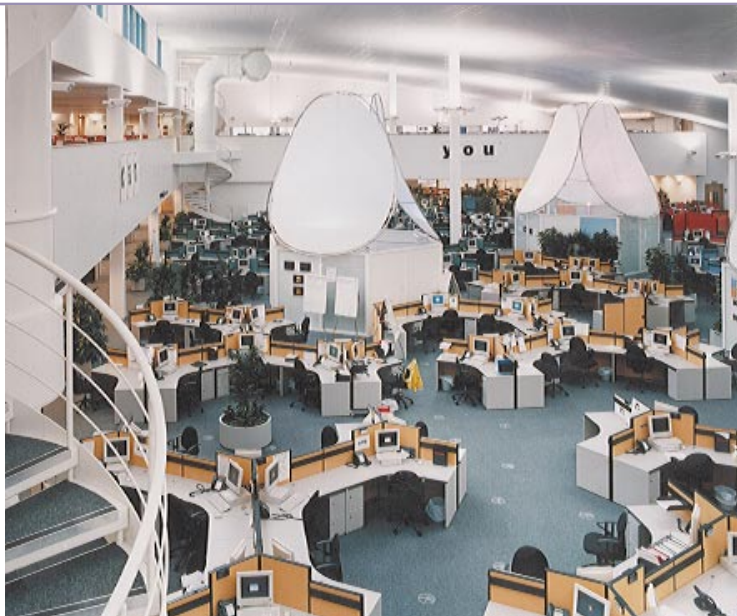
Shepherd Engineering Services has recently completed this £1.4 million m&e contract for call centre client Orange. The new 7000 m 2 customer services centre in Tyneside is designed to accommodate up to 1000 employees.
